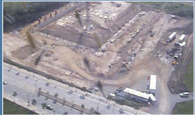
Construction is underway at the site of the new Niagara Convention and Civic Centre in Niagara Falls. Local officials celebrated the milestone with a groundbreaking ceremony on May 1, 2009.
